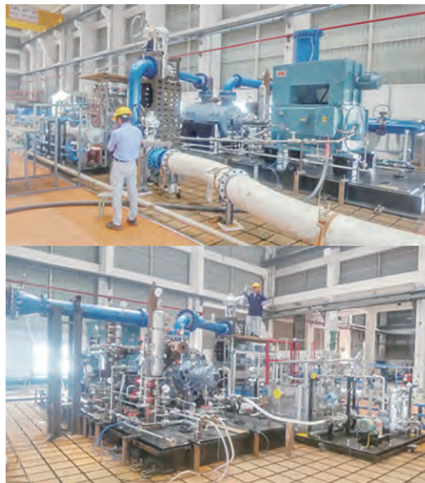
図7 DCIPL社での試運転 Fig.7 Test at India Factory
