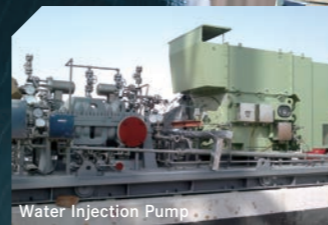
Water Injection Pump
