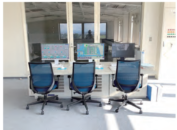
図6 監視操作設備外観 Fig.6 View of Supervisory control panel
