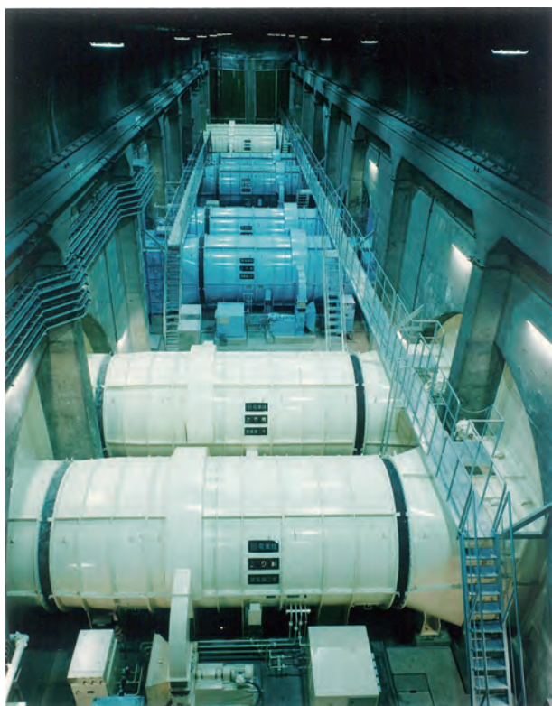
図1 関越トンネル換気用送風機外観 (1) Fig.1 View of Kan-etsu Tunnel ventilation fans
