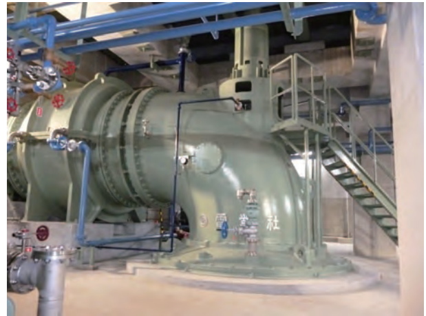
図3 No.5雨水ポンプ外観 Fig. 3 No.5 View of pump
