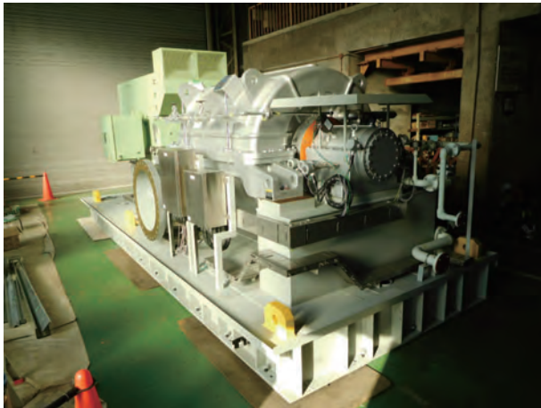
図4 Main Air Blower外観 Fig.4 View of Main Air Blower
