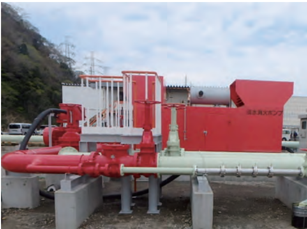
図4 消火ポンプ設備 Fig.4 View of fire water pump station
