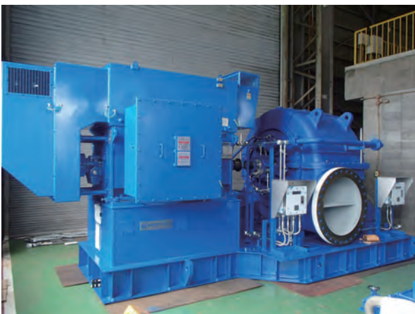
図3 Incinerator Air Blower 外観 Fig.3 View of Incinerator Air Blower
