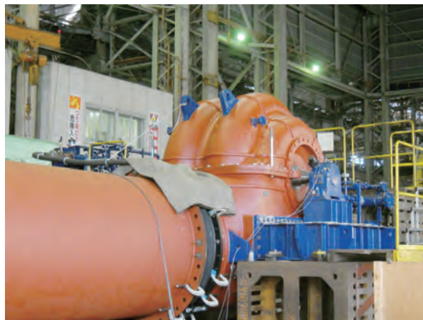
図3 Main Air Blower外観 Fig.3 View of Main Air Blower
