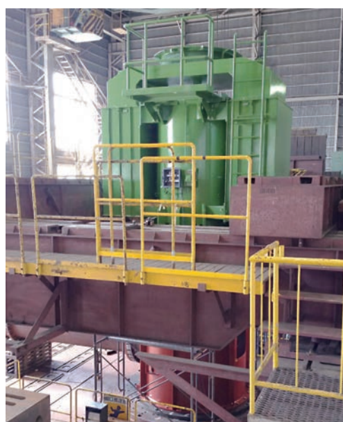
図10 Circulating water pump
