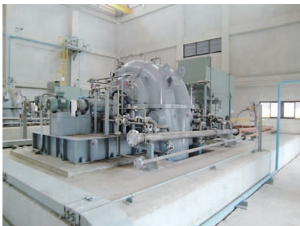
図9 ブロワ現地据付状態 Fig.9 View of blower at site
