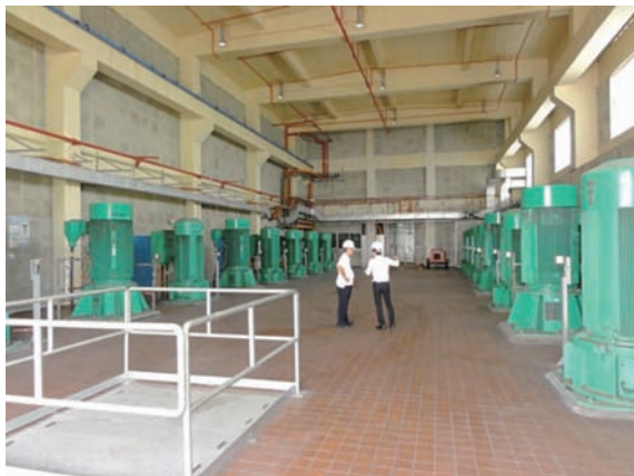
図4 汚水ポンプ設備 (モータ室) Fig.4 Sewage pump equipment (Motor floor)
