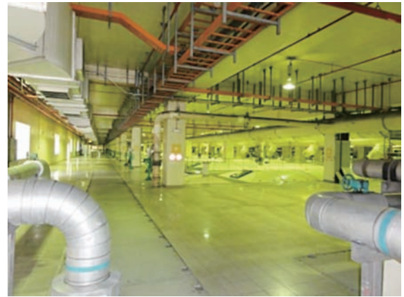
図6 反応層設備 Fig.6 Reaction tank equipment
