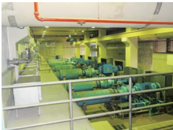
図5 曝気ブロウ設備 Fig.5 Aeration blower equipment
