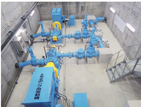
図3 揚水ポンプ据付外観 Fig.3 View of installed pumps installed
