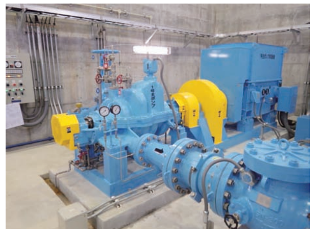
図5 揚水ポンプ外観 Fig.5 View of pump
