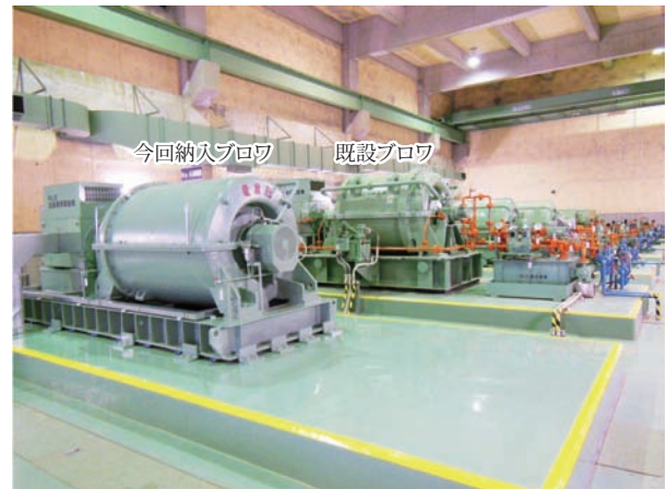
図6 機場写真 Fig.6 View of blower station
