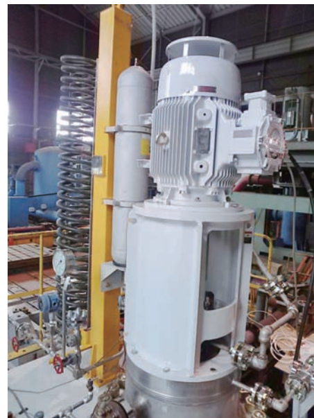
図7 Condensate transfer pump
