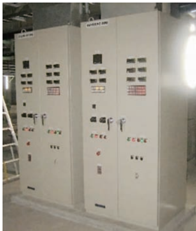
図6 動力制御盤 Fig.6 View of power operator control panel
