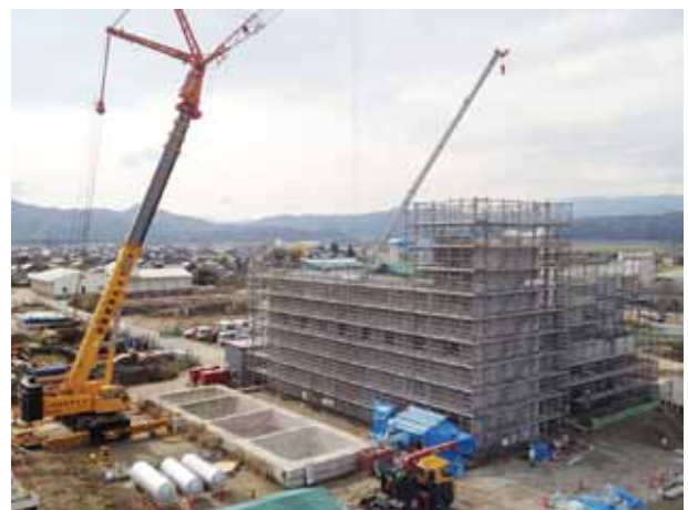
図7 ポンプ据付状況 Fig.7 View of pump installation by 300 t class crane
