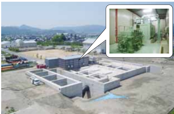
図6 仮設上屋とNo.1ポンプ設備 Fig.6 A temporary housing & No.1 pump equipment
