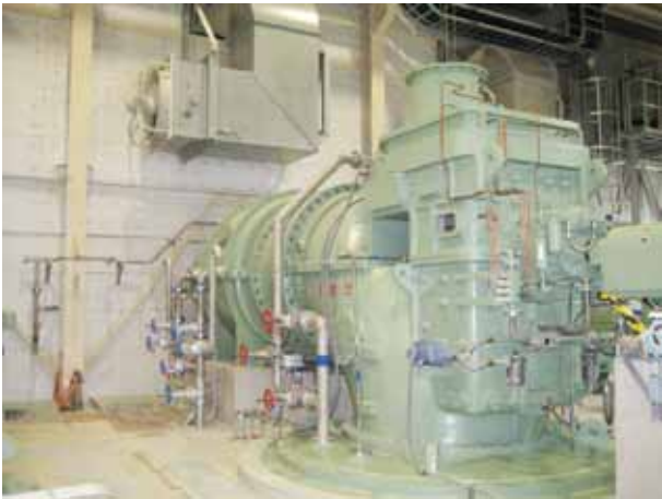
図1 1号主ポンプ Fig.1 View of No.1 pump
