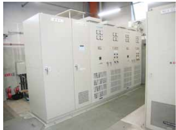
図4 吐出し弁用制御盤および直流電源盤 Fig. 4 Discharge valve control panel and DC power supply
