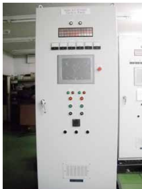
図7 制御盤 Fig.7 View of UCP
