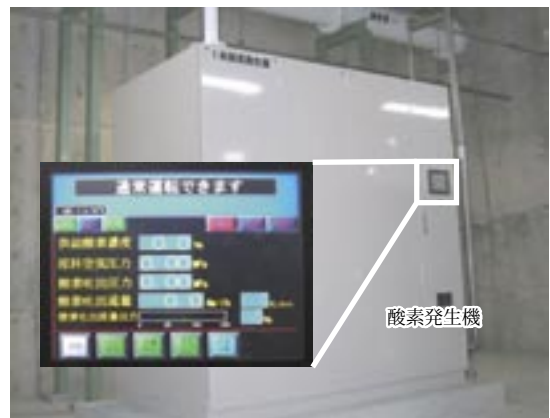
図11 酸素発生機 Fig.11 View of oxygen generator
