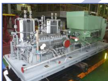
Water Injection Pump
