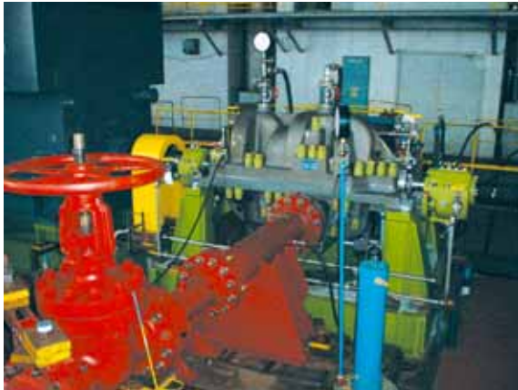
図4 社内試運転 Fig. 4 Shop performance test
