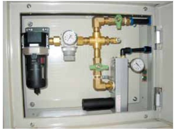
図4 装置内機器配置 Fig. 4 Equipment layout of apparatus inside
