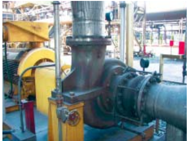
図19 ガス冷却水ポンプ現地据付状況外観 Fig.19 View of gas cooling water pump at site
