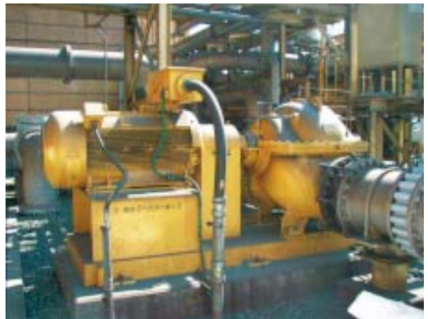
図16 海水ブースターポンプ現地据付状況外観 Fig.16 View of sea water booster pump at site
