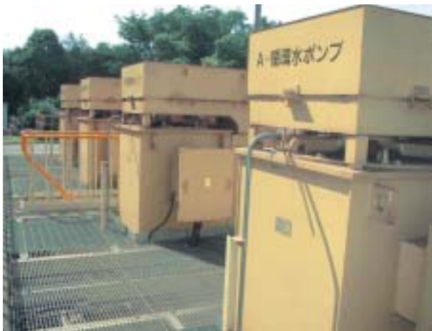
図7 循環水ポンプ現地据付状況外観 Fig. 7 View of CWP at site
