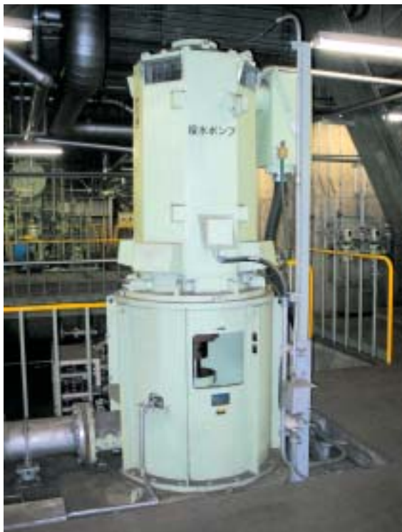
図10 復水ポンプ現地据付状況外観 Fig.10 View of CP at site
