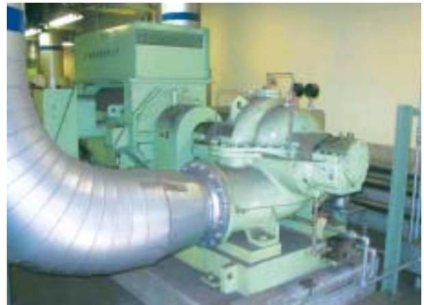
図13 軸受冷却水ポンプ現地据付状況外観 Fig.13 View of bearing cooling water pump at site
